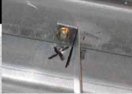
HVAC Duct Strap
